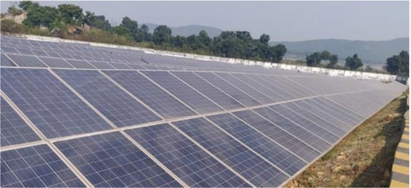
Figure 1 Ground Mounted Solar panels in MCL
